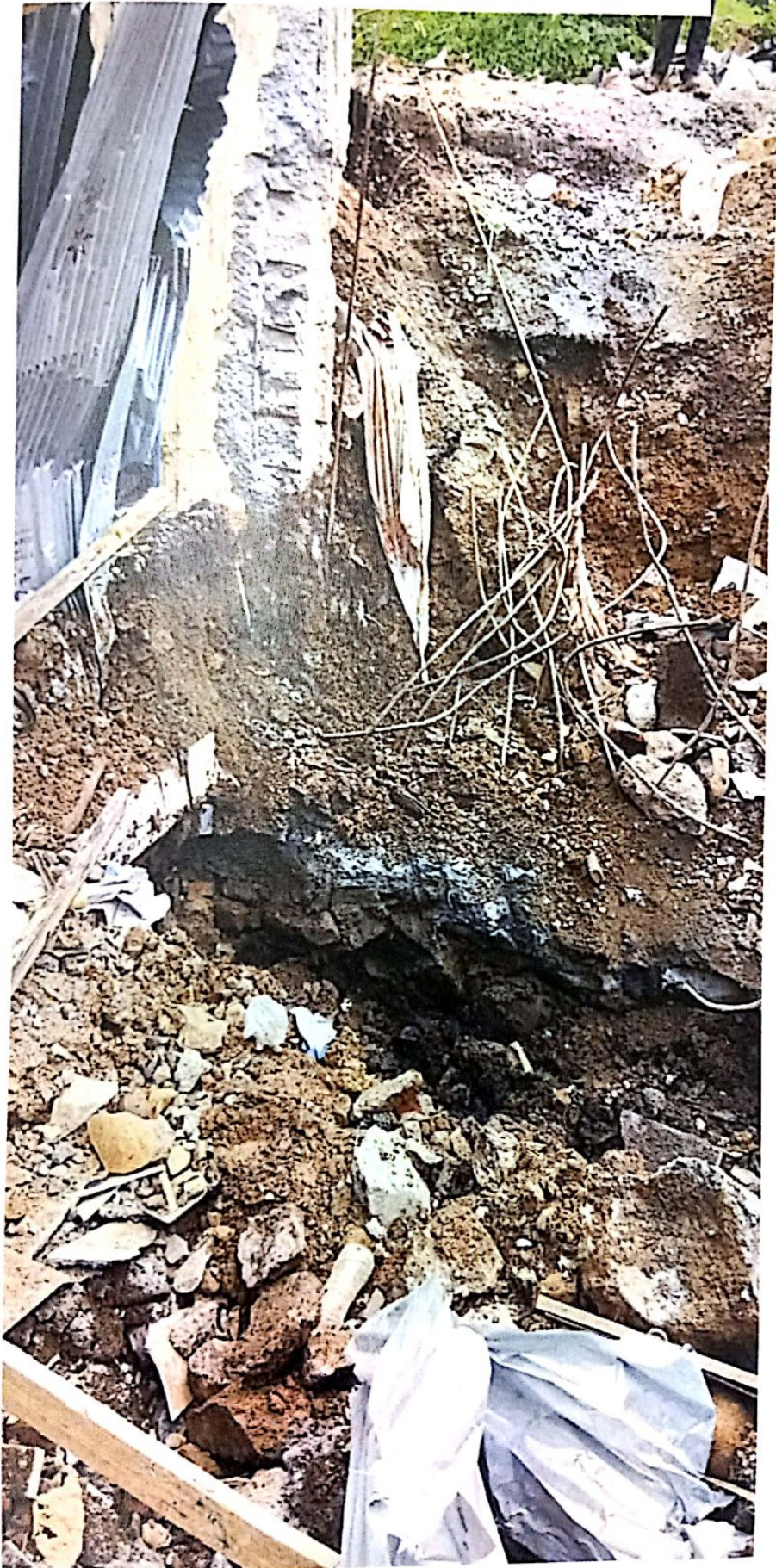
Excavation beneath the wall foundation to ascertain the scouring if any at Pimripada
